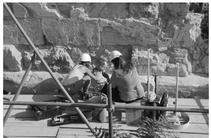
Conservation works on the north Acropolis wall, B12 area. Photo A. Tsimereki, 2021
