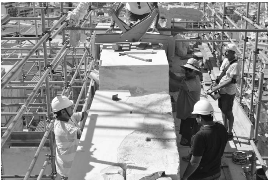
Trial positioning of a stone block of the backing wall of the Parthenon's west pediment. Photo K. Skaris, 2022.
