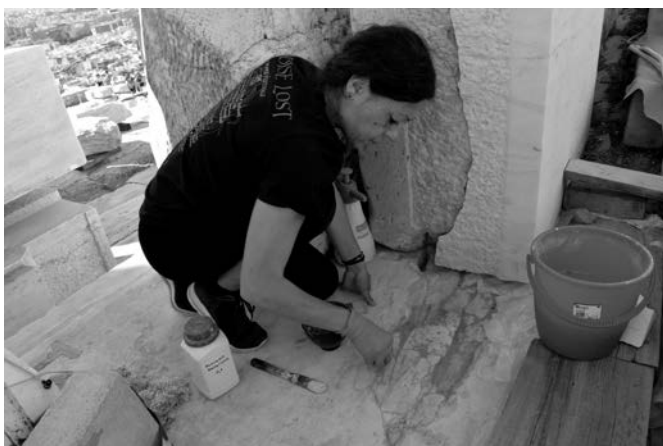
Conservation of the toichobate blocks of the south wall of the Parthenon cella. Photo S. Gabrielidou, 2022
