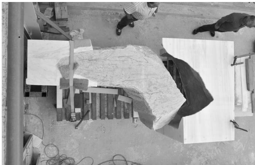
Adjusting a new marble addition for the Parthenon's orthostate, northeast parastasis. The addition was created in CNC with digital scanning of the mould. The "mixed method." Photo V. Manidaki, 2014
