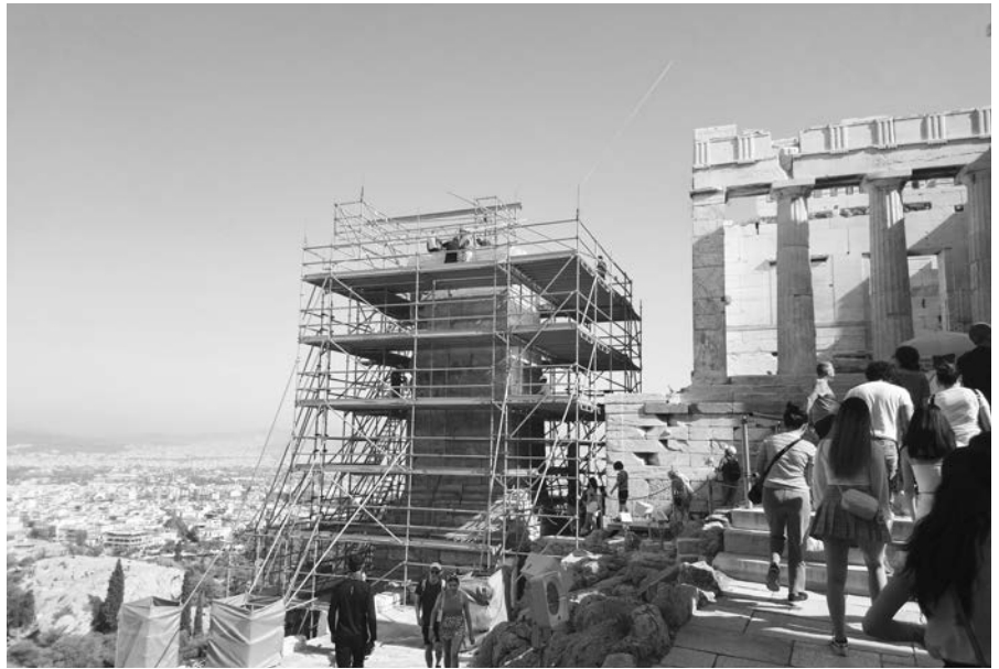
View from the S after the scaffolding was mounted to the crown of the Pedestal. Photo V. Eleftheriou, 2022
