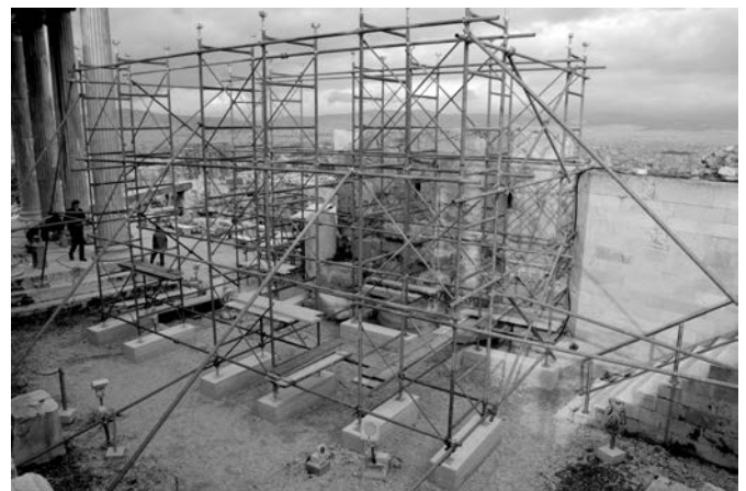
Setting up a scaffolding for the commencement of works in the B12 area of the Acropolis north wall. Photo V. Eleftheriou, 2022
