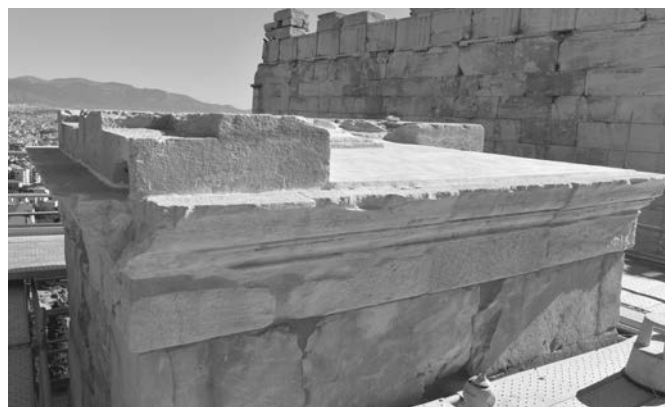
View from the S of the monument's superstructure after conservation and the restoration of the crown's waterproofing. Photo K. Frantzikinaki, 2022
